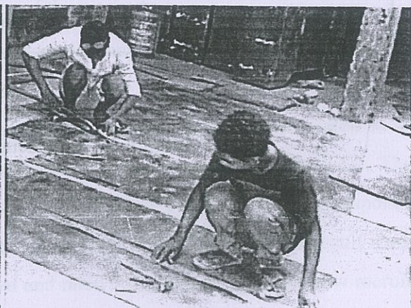
Figure 12: sharp edges exposed to hands and feet
